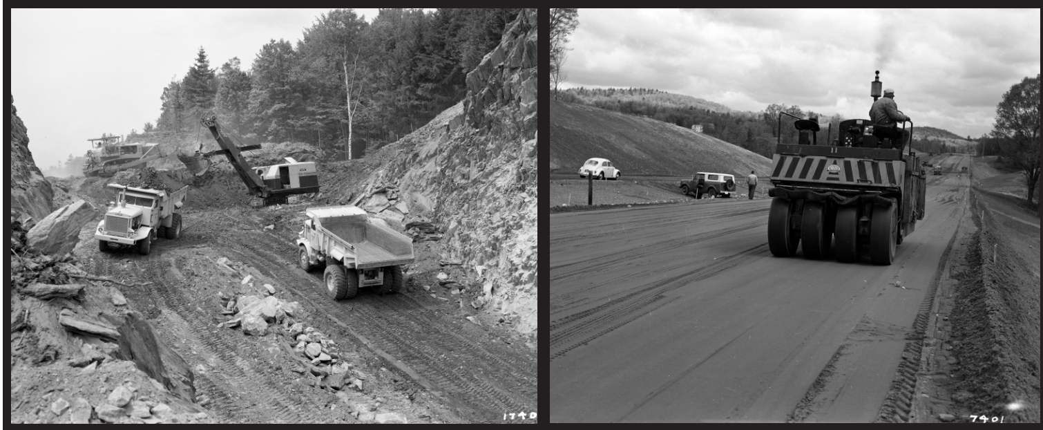
Figure 5. Interstate excavation and preparation for paving. The image to the left was taken in 1959, and is of excavation and interstate construction near Montpelier, Vermont. The image to the right was take in 1963, and shows men using machinery to flatten the road for future pavement near Westminster, Vermont. These images were sourced from the Landscape Change Program database (LS37392_000/LS41753_000).
